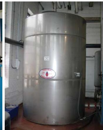
A hot water storage tank in the plant.
