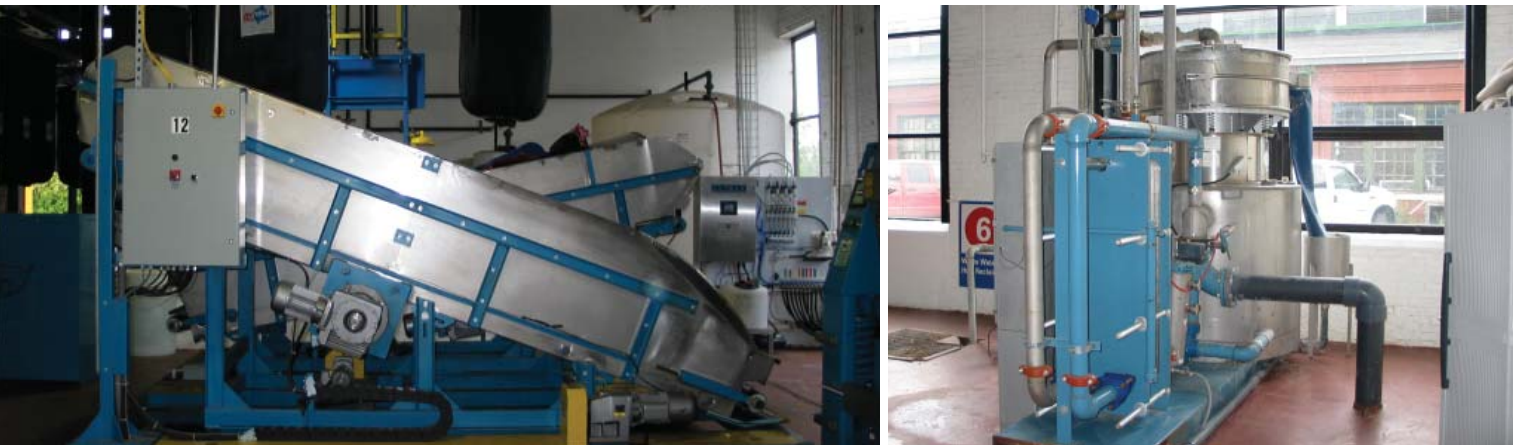
A shuttle system in the wash aisle moves goods from the washer/extractors to the dryers. Another view of the heat reclaimer and shaker screen equipment
