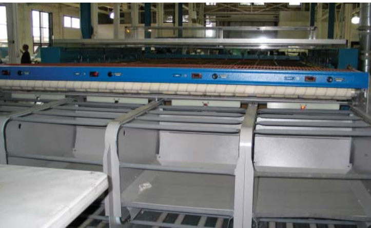
Small piece stacking equipment at the back end of an ironer
