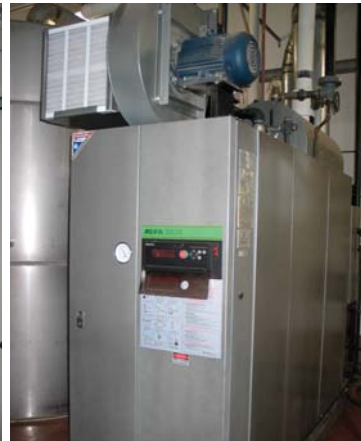
One of three 100 HP Miura boilers save energy by heating up quickly when needed and powering down when demand drops.
