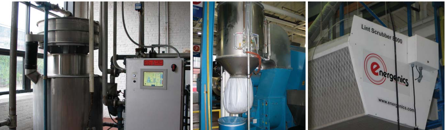
(l/r) A view of shaker screen equipment for removing impurities from wastewater and a heat-recovery system A lint-collection system in the wash aisle This equipment filters air in the plant to remove lint.
